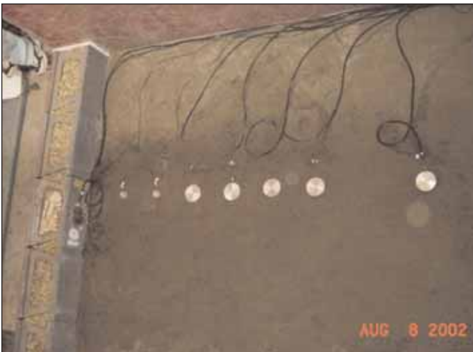
Load Transducers for Measuring Vertical Earth Pressure
